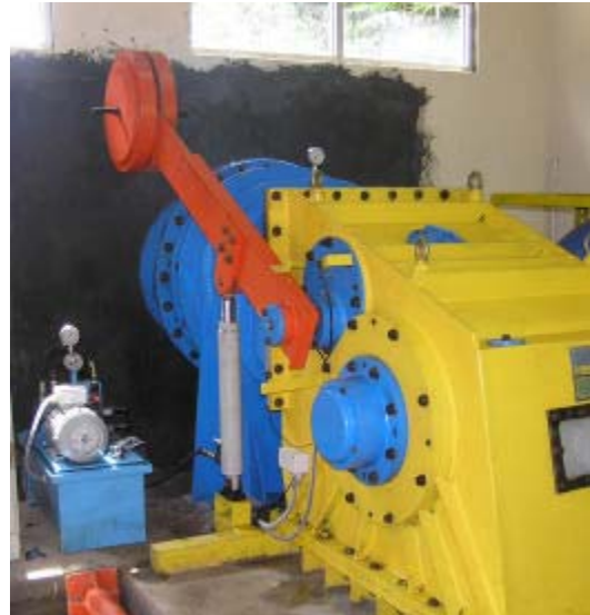
Turbine Actuator for T-14
